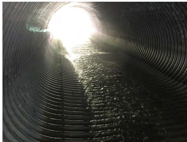
Deformation on culvert floor at midspan
